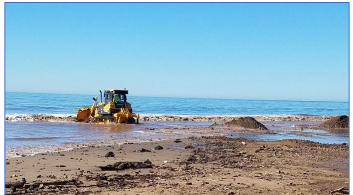
Photo of dumping debris from petition website. Photo is by the Army Corp of Engineers.
