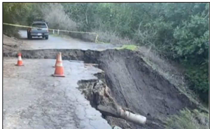
Above: the access road to the Sequoians club is washed away.
